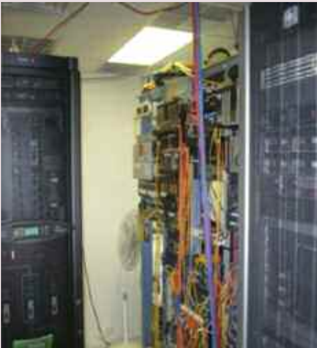
Figure 3. Cramped, inefficient, out of data IT shed.
